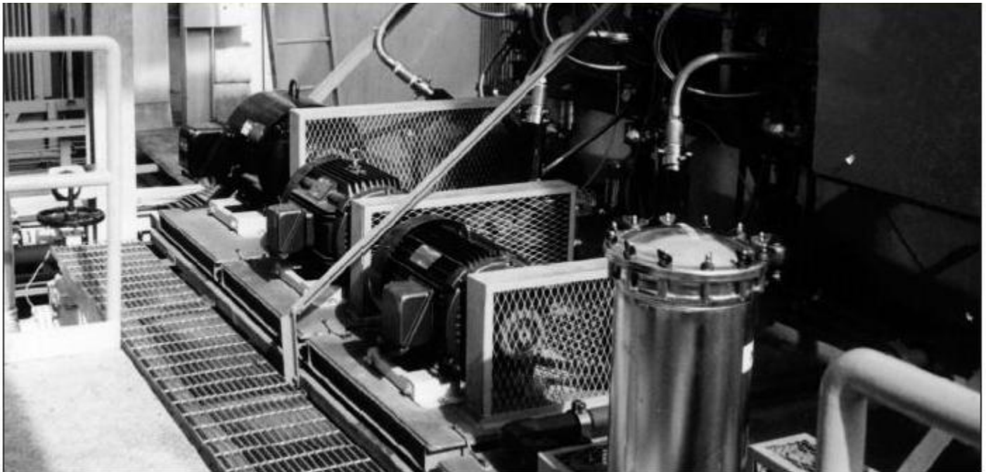
Fig. 8: Pump skid to supply demineralized water to the external, internal and overspray zones for W501B5.
