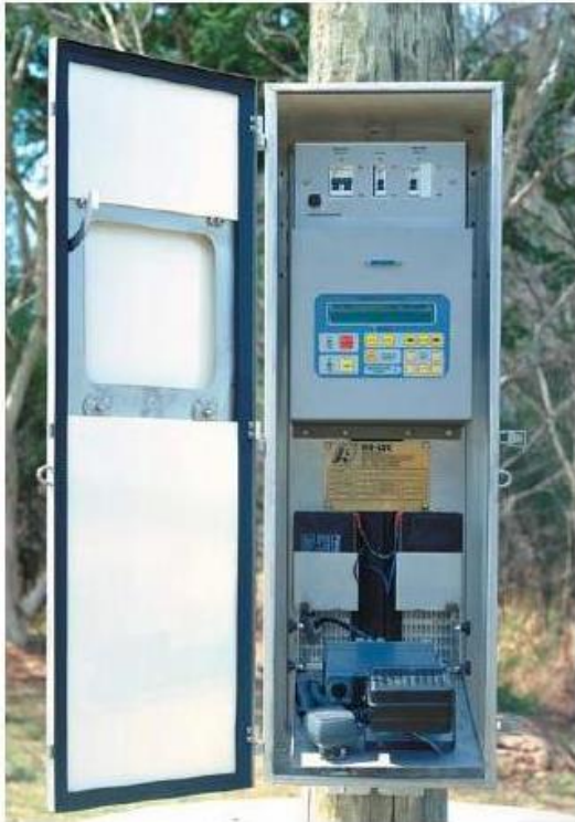
Pole Top Control & Communications Cubicle
